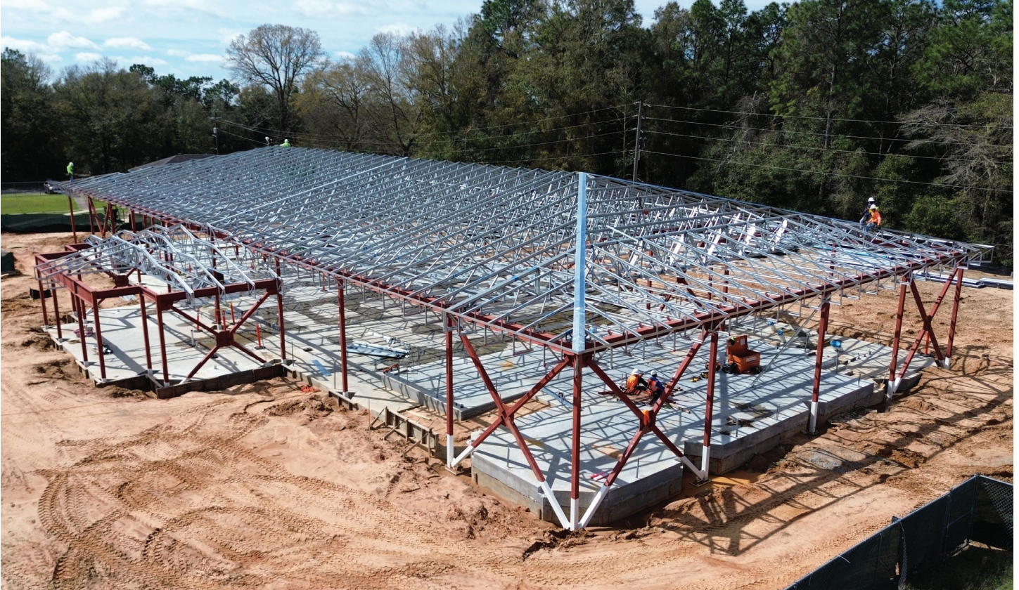
Alpine® TrusSteel project featuring 79 ft.-10 in. span.
