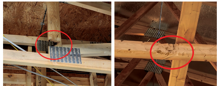
Figure 1. Two install examples of poor-quality lumber that impacted the integrity of truss members.
