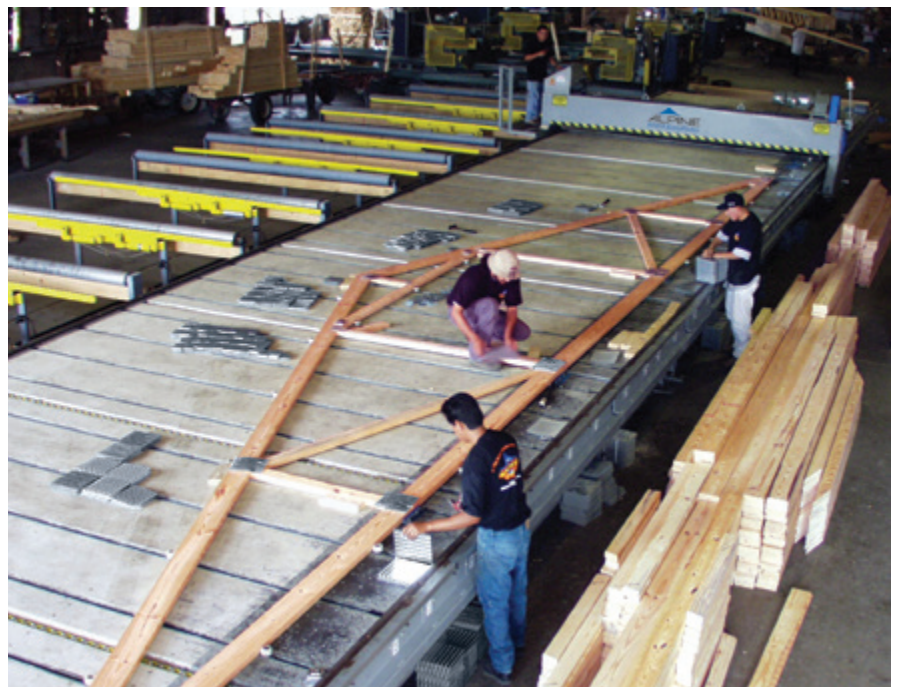
Without walkways, the entire working surface can be used for jigging and pressing. The gantry operator steps from the platform directly onto the table to position the upper truss pieces and connectors.
